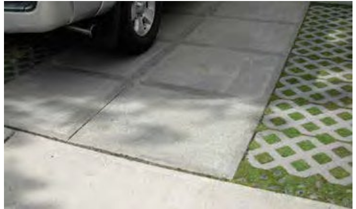
Cast-in-place concrete and permeable unit pavers
